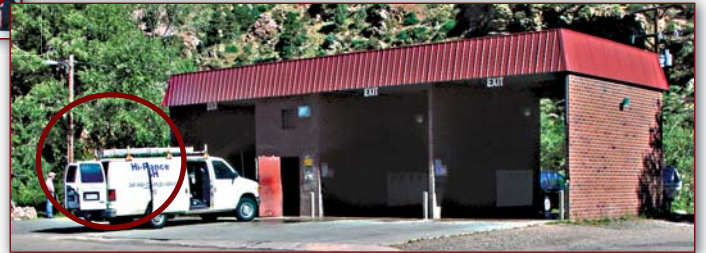
Exit side of the car wash before the remodel. Circled area shows where the automatic will be built.
