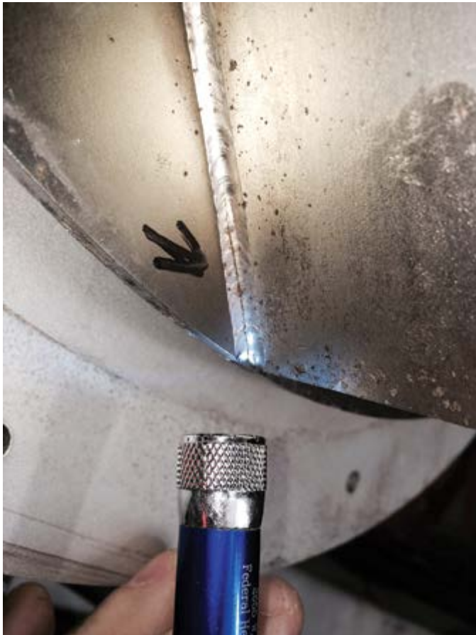
The arrow is pointing to the stress fracture in this blower impeller.
